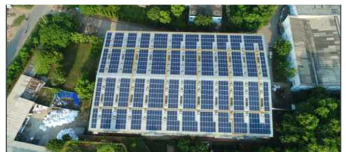
Solar panels on the roof top of the Baddi unit
