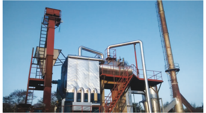
New boiler at the plant
