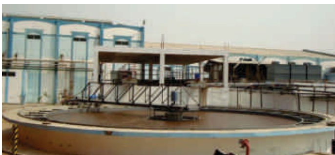
The upgraded ETP at the Sara Textiles plant in Nalagarh
